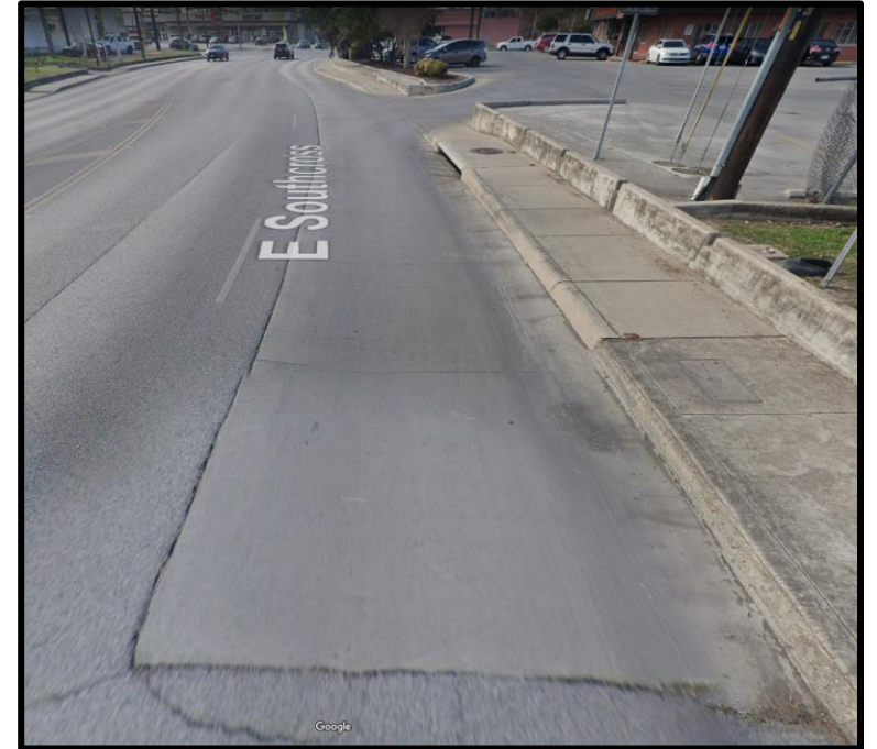
Facing west on E. Southcross. Concrete VIA bus pad (to remain) on westbound lane shown.
